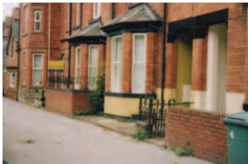
Unightly repairs and alterations
