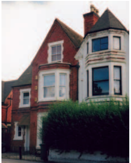
Unsightly painted brickwork
