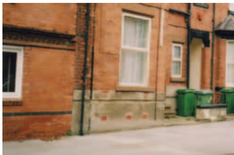
Unsympathetic repairs and alterations
